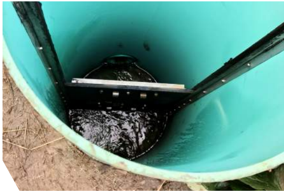
Outlet Control Structure
