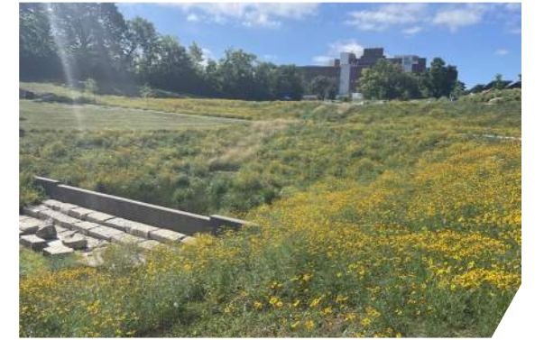
Overflow Surface Weir
