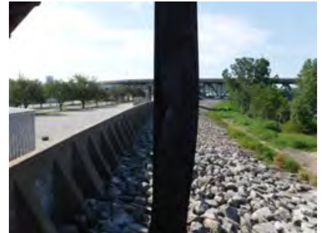
impact damage to LI-UI on span 3
