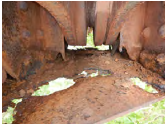
typical loss in secondary member
