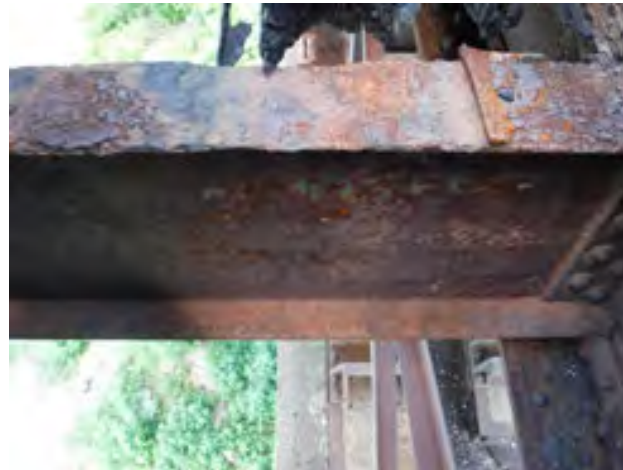
typical loss to stringer top flange
