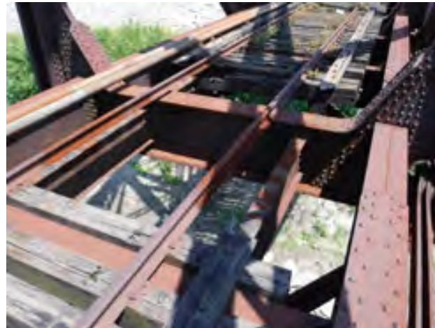
missing bridge ties from fire
