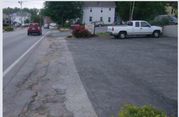
Fig. 3.17 – Example of the lack of sidewalk connectivity that plagues Downtown Parkville.
